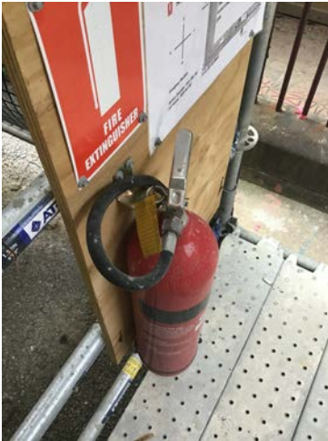
BLD C Level 1 Scaffold - FE tag without any inspection mark.
