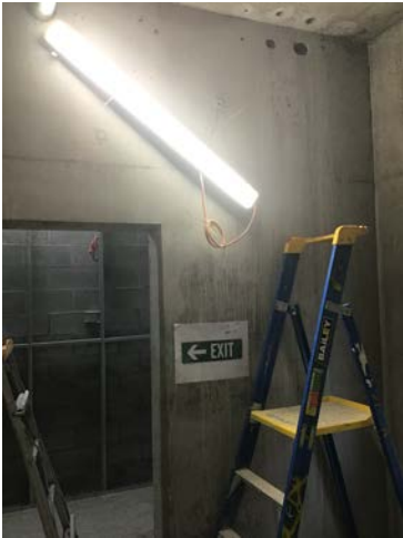
BLD C Level 1 - Stair C2 Temp Light
