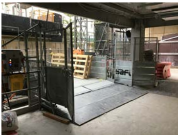
BLD C Hoist - Materials left in the hoist, gate open, no operator manning hoist
