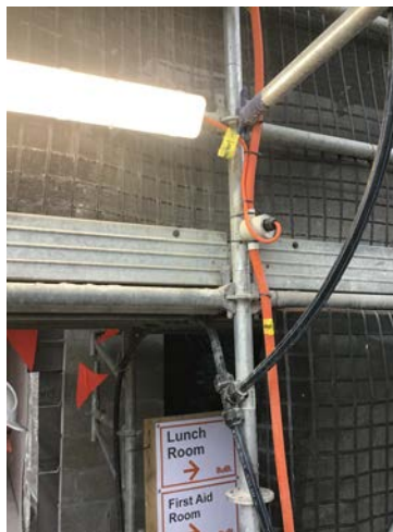
Level 2 temp light cable unprotected.
