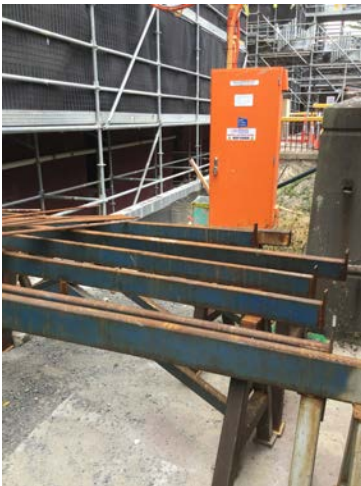
Temp MSB access blocked.
