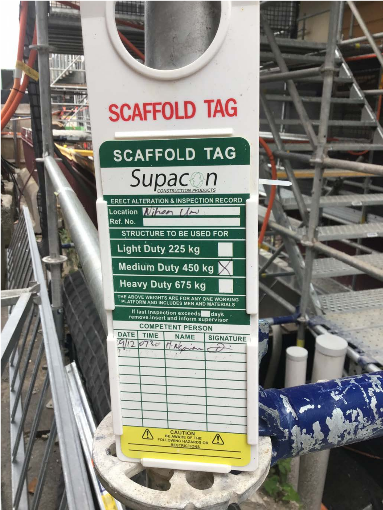
Scaffold tag current
