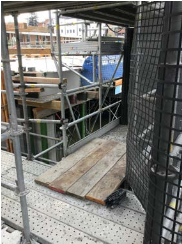
BLD A Level 4 North East Facade - Block off access or install screens to prevent falling objects below.
