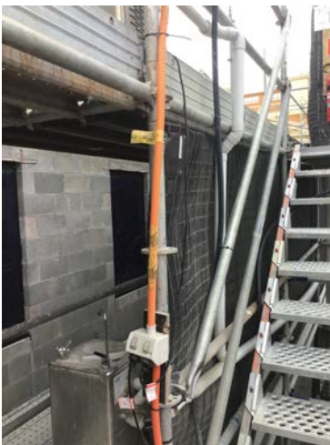
Level 4 bubbler lead unprotected.
