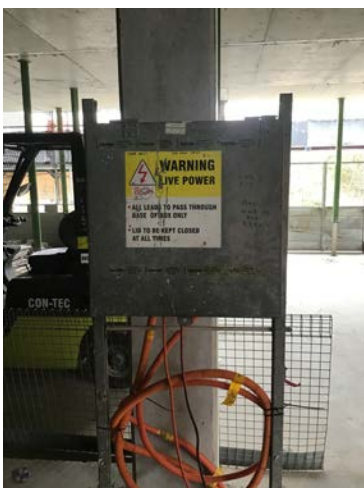
BLD A Level 2 temp switchboard
