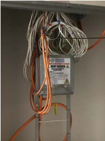
BLD C Level 1 DB Cupboard & Temp DB
