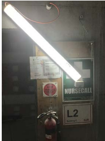
BLD C Level 2 - Stair C2 Temp Light
